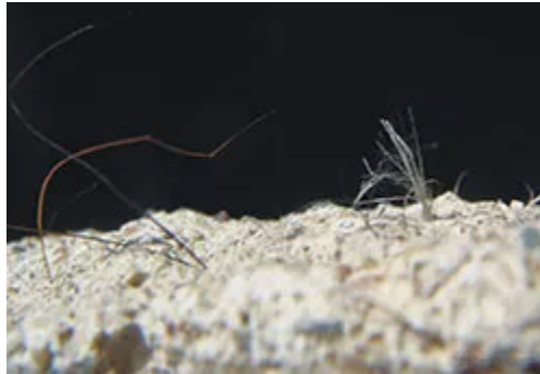
Drilling into drywall containing asbestos will release fibers into the air.
