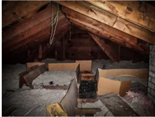
Attic insulation in older homes may contain asbestos that could fall through ceiling cracks.
