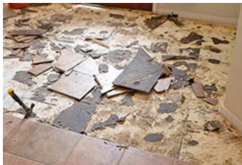
Loose vinyl tiles can expose asbestos-containing adhesive.
