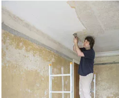
Scraping a popcorn ceiling containing asbestos can be hazardous without proper masks and ventilation.
